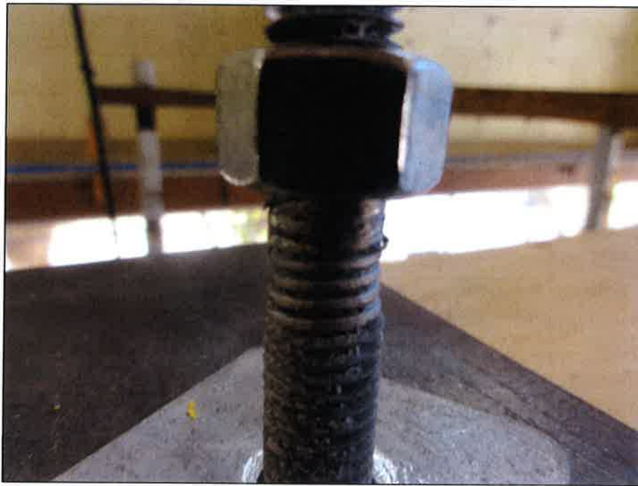
Figure 6: Photograph of Tie-Down Rod after Failure
